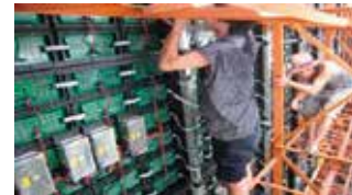
Difficult to maintain, High maintenance costs.
